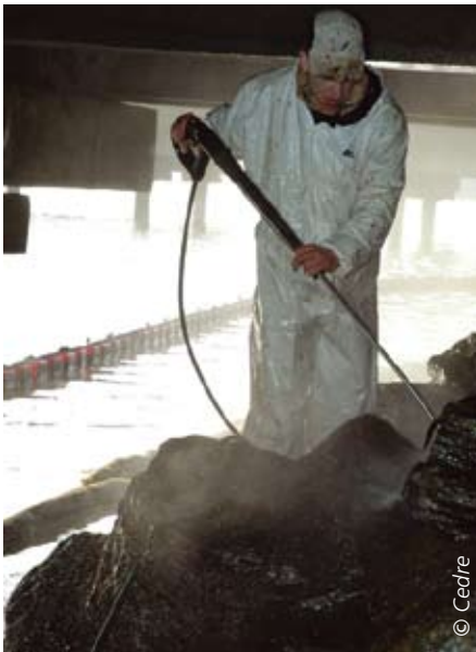
Cleaning riprap under a wharf on piles in a port with a large tidal range.
